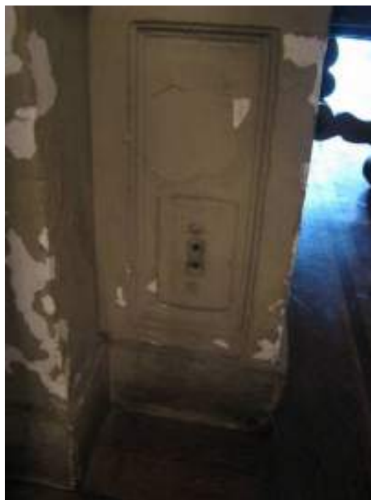
43-PERDIDA DE RELIEVE-RAYADURA
