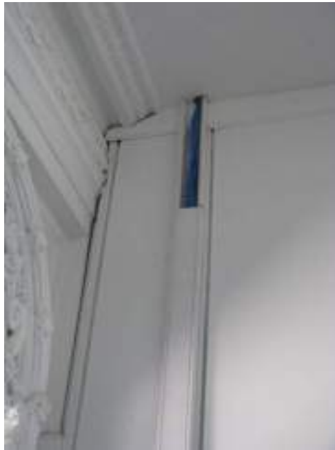
42-INSTALACION NO ORIGINAL-PERDIDA DE RELIEVE
