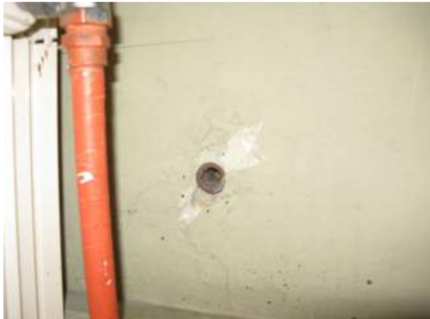
15-INSTALACION NO ORIGINAL-PERFORACION
