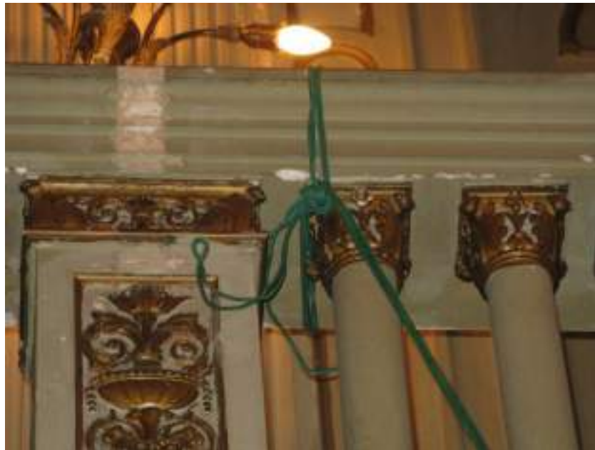
11-INSTALACION NO ORIGINAL-RAYADURAS
