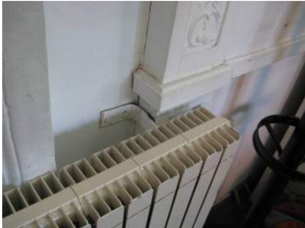
16-FISURAS-INSTALACION NO ORIGINAL
