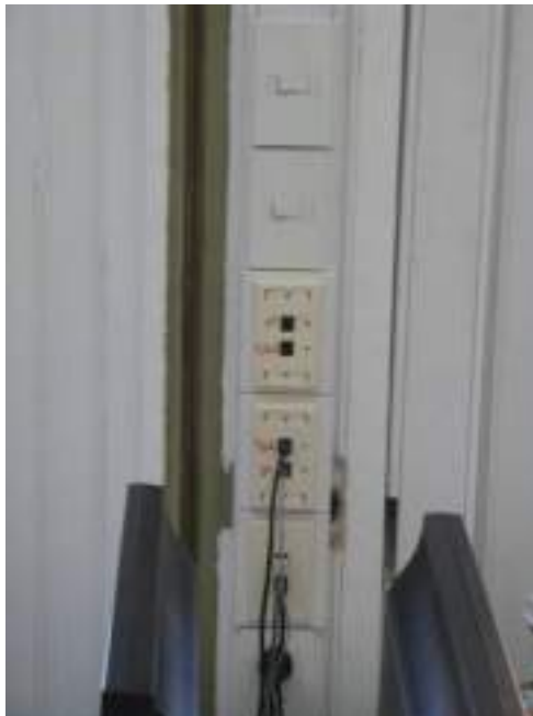
51-INSTALACION NO ORIGINAL-PERFORACIONES
