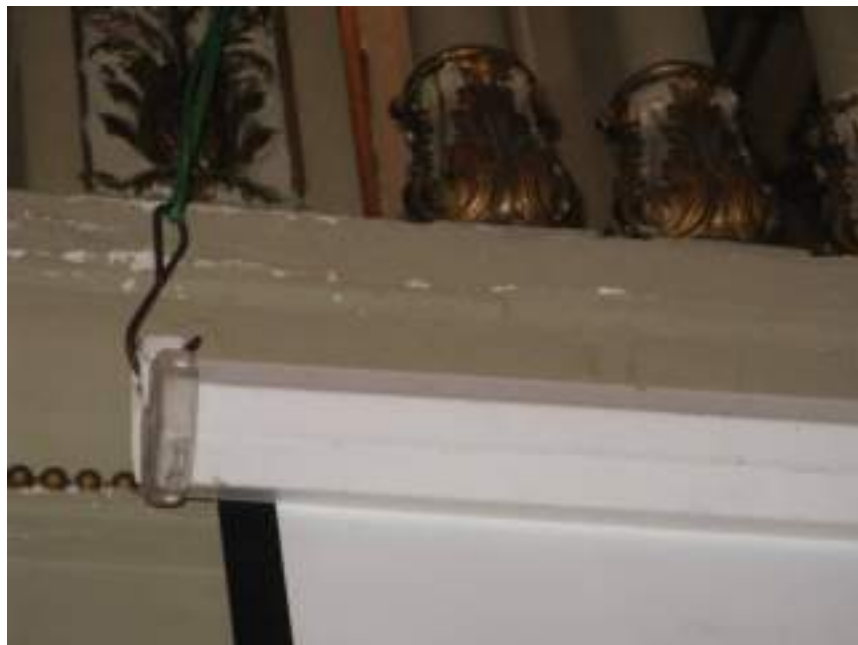
4-INSTALACION NO ORIGINAL-FISURAS
