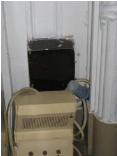
49-INSTALACION NO ORIGINAL-PERFORACION
