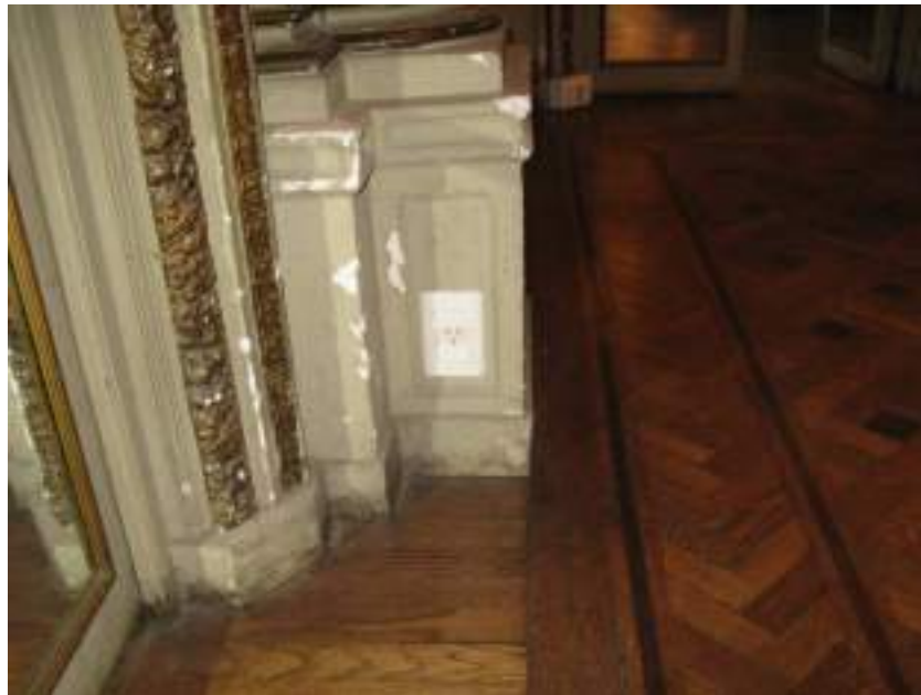
85-FALTANTE PARCIAL-INSTALACION NO ORIGINAL-RAYADURA
