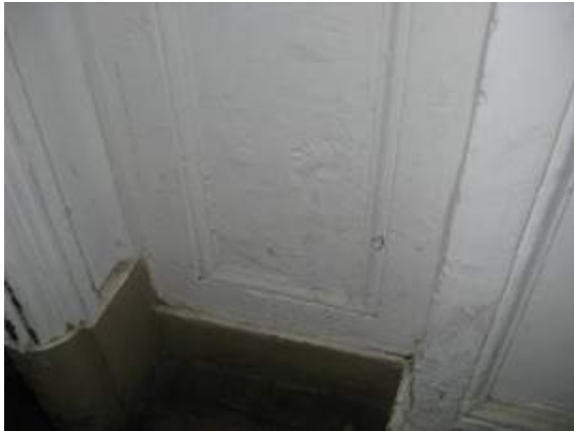
4-PERDIDA DE RELIEVE-RAYADURA
