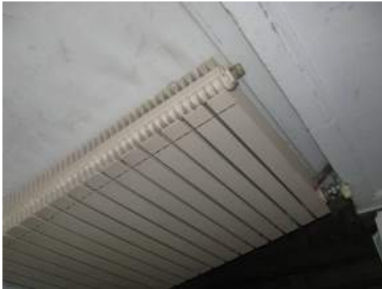
34-INSTALACION NO ORIGINAL-PERDIDA DE RELIEVE
