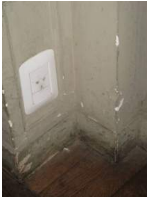
89-INSTALACION NO ORIGINAL-PERDIDA DE RELIEVE-RAYADURA
