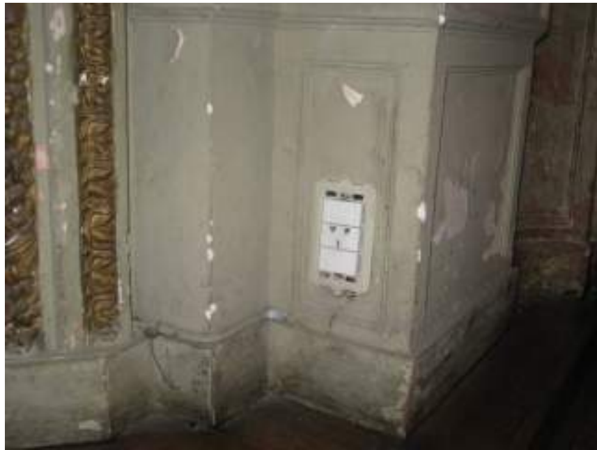
27-INSTALACION NO ORIGINAL-PERDIDA DE RELIEVE-RAYADURA
