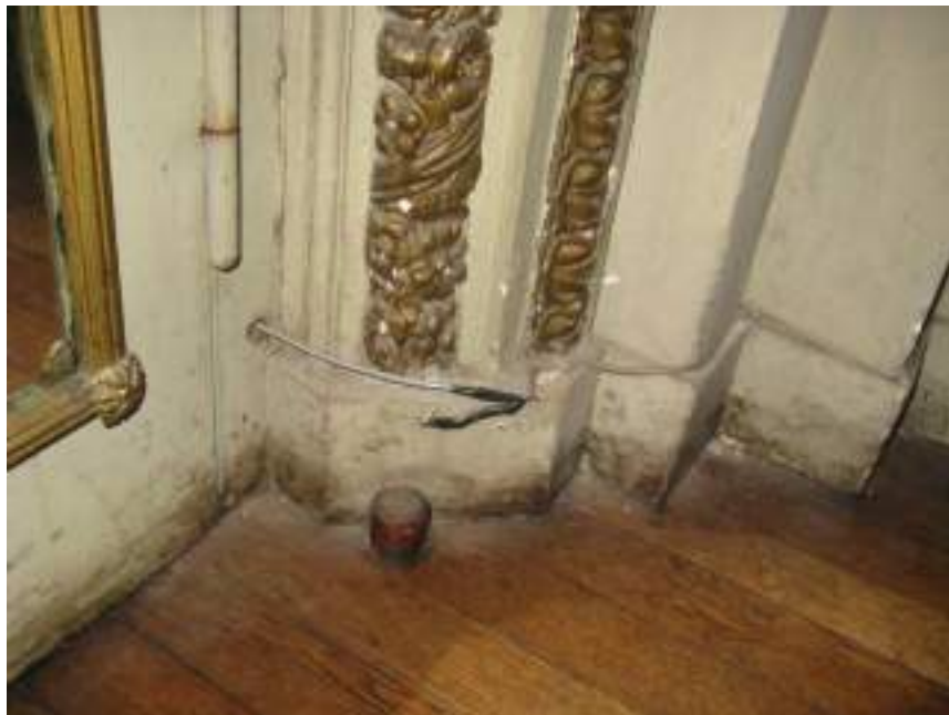
62-INSTALACION NO ORIGINAL-PERDIDA DE RELIEVE-RAYADURA
