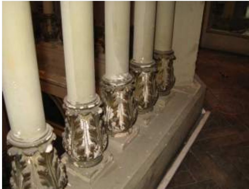
3-CAPA PICTORICA DISGREGADA-INSTALACION NO ORIGINAL
