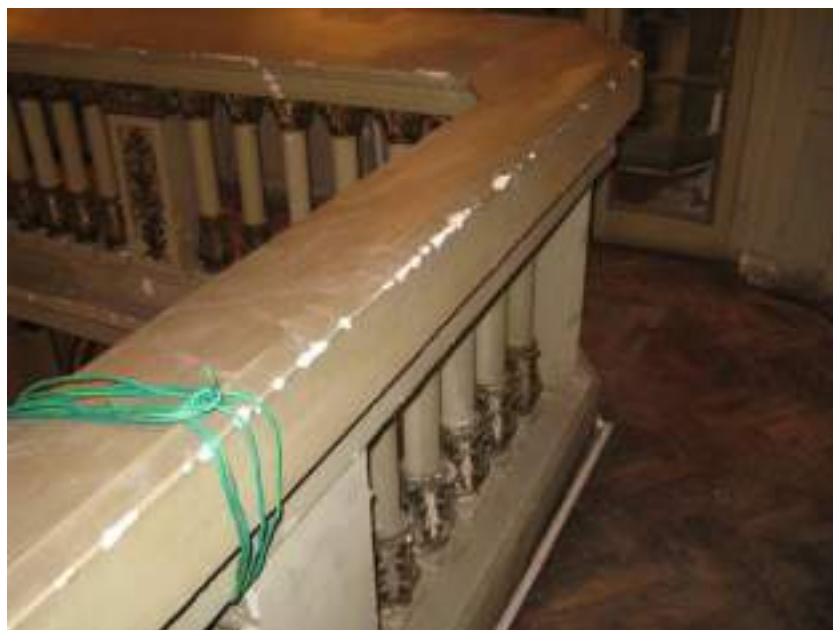
6-INSTALACION NO ORIGINAL-PERDIDA DE RELIEVE-RAYADURAS
