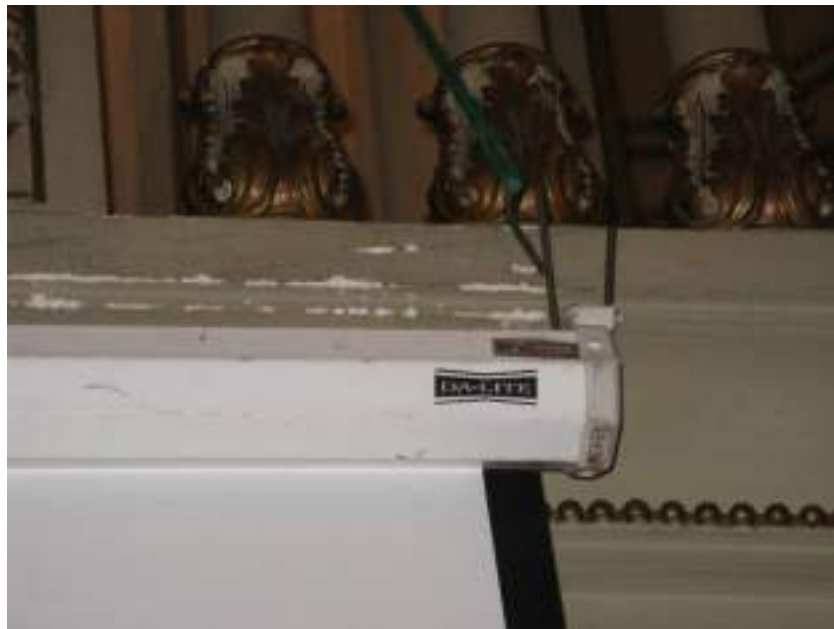
10-INSTALACION NO ORIGINAL-RAYADURAS
