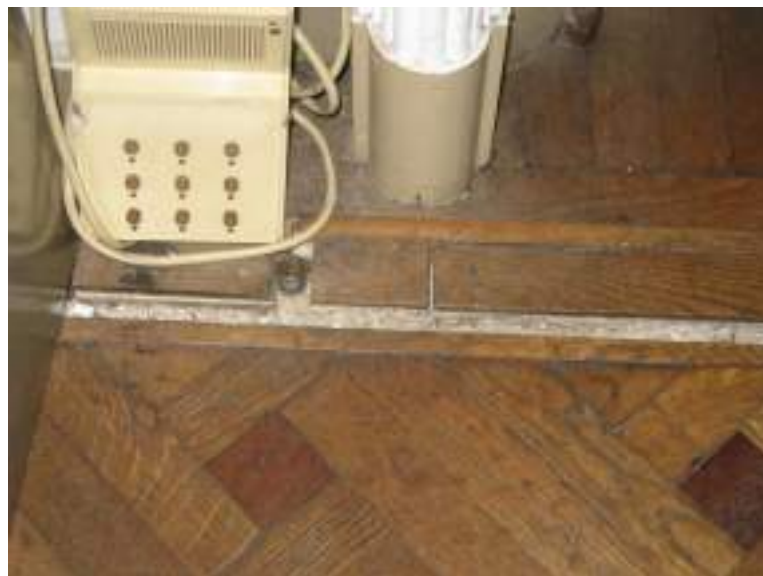
45-INSTALACION NO ORIGINAL-FALTANTE TOTAL
