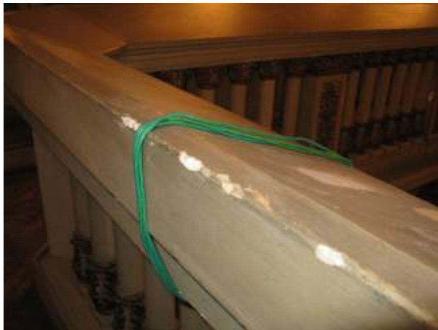
12-INSTALACION NO ORIGINAL-PERDIDA DE RELIEVE
