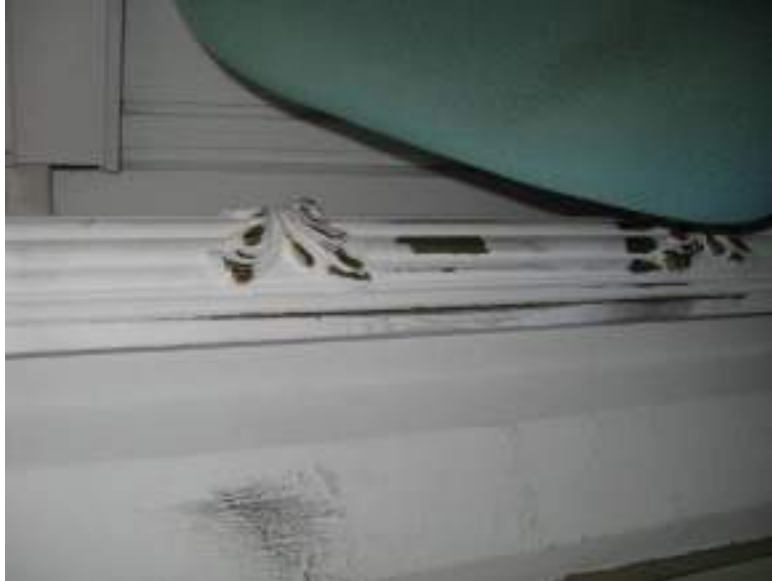
46-PERDIDA DE RELIEVE-RAYADURA
