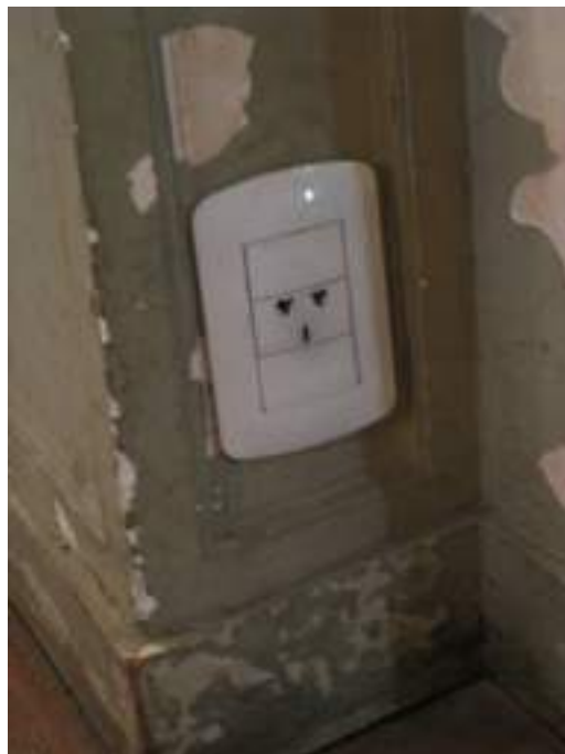
18-INSTALACION NO ORIGINAL-PERDIDA DE RELIEVE
