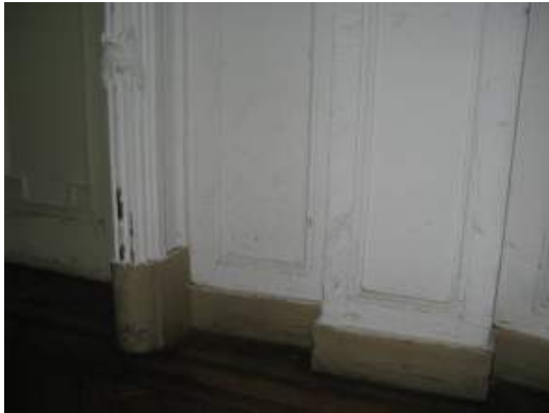
5-PERDIDA DE RELIEVE-RAYADURA
