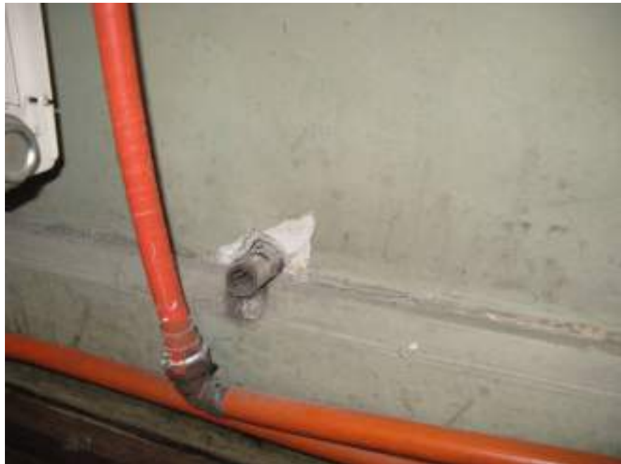
17-FISURAS-INSTALACION NO ORIGINAL-PERFORACION
