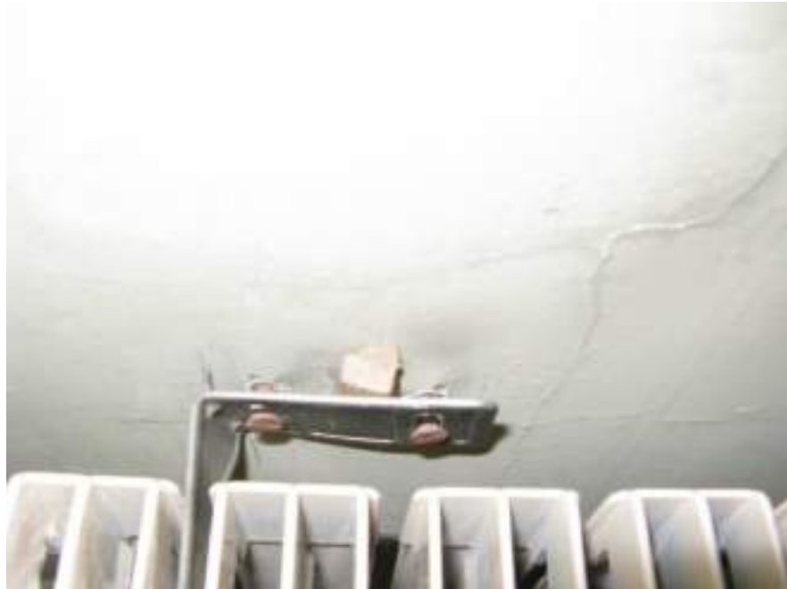
20-INSTALACION NO ORIGINAL-FISURAS-PERFORACION
