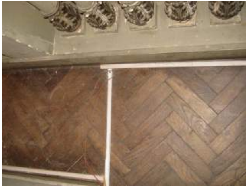
17-PA-INSTALACION NO ORIGINAL-PERFORACIONES
