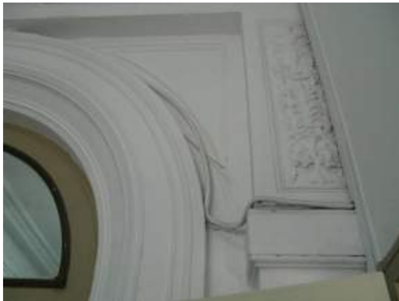
7-INSTALACION NO ORIGINAL
