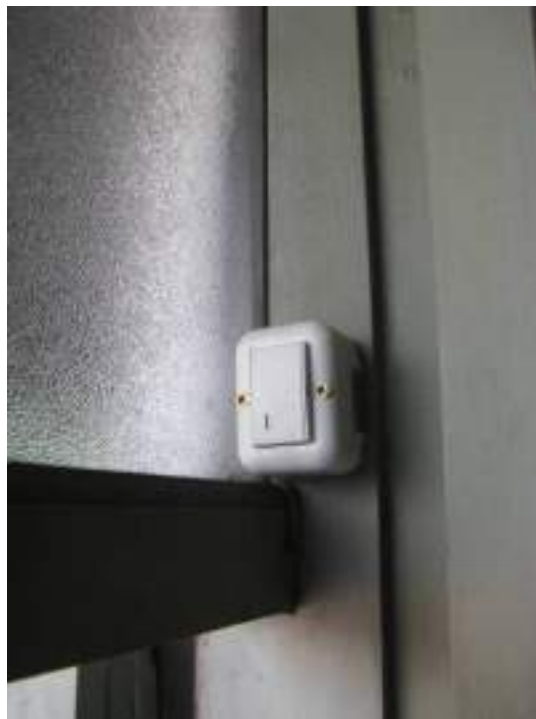
52-INSTALACION NO ORIGINAL
