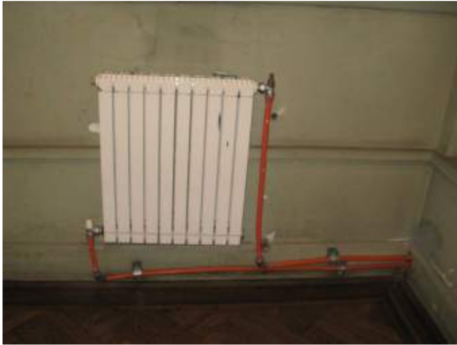
18-FISURAS-INSTALACION NO ORIGINAL-PERFORACION
