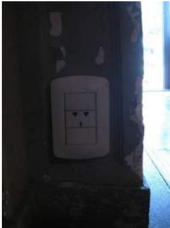
41-INSTALACION NO ORIGINAL
