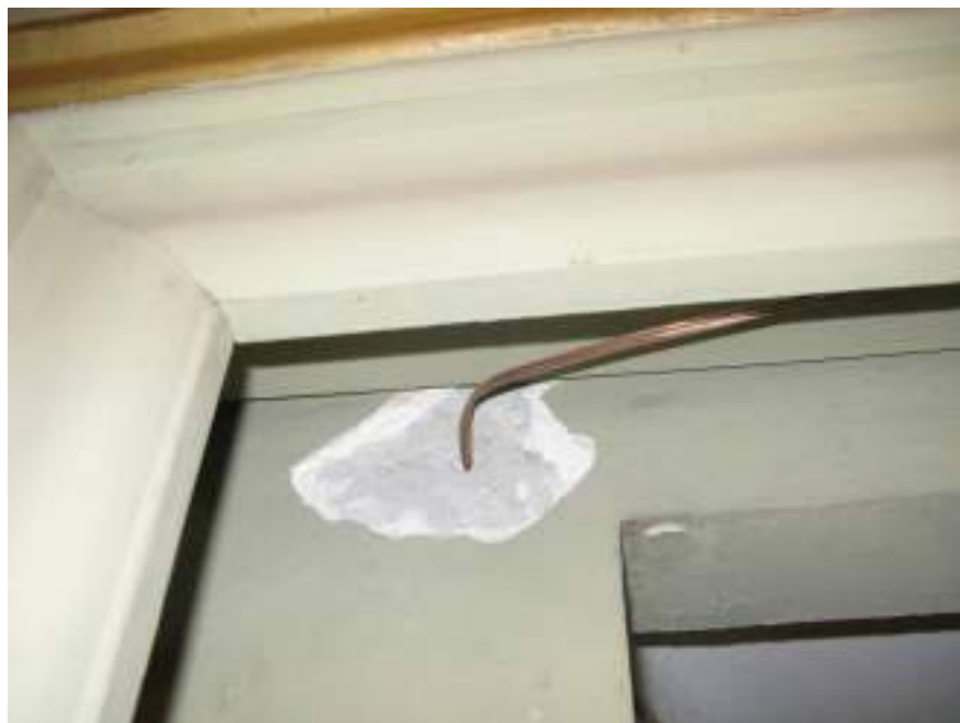
33-INSTALACION NO ORIGINAL-PERFORACION
