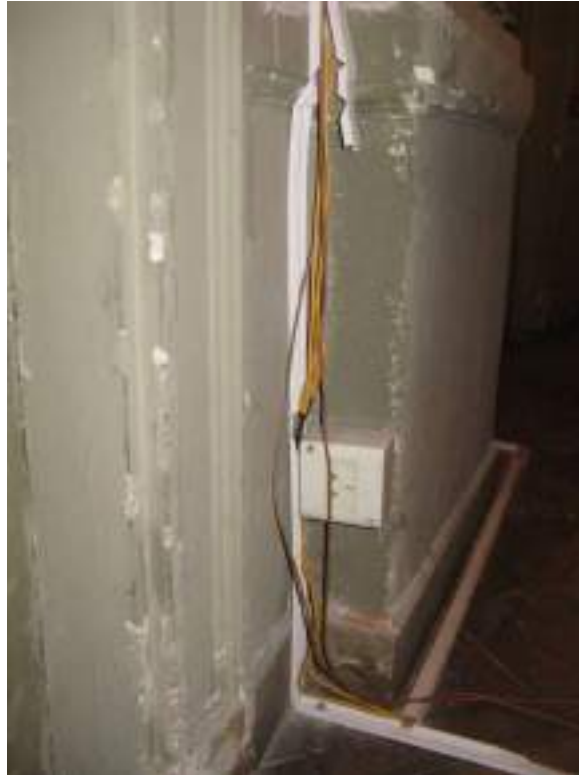
14-INSTALACION NO ORIGINAL-PERDIDA DE RELIEVE
