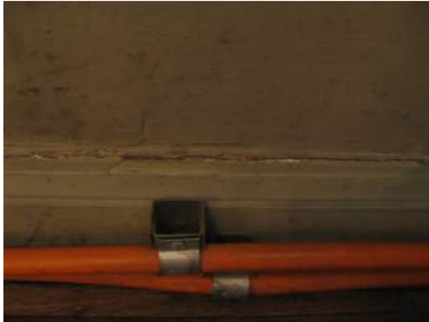
16-FISURAS-INSTALACION NO ORIGINAL
