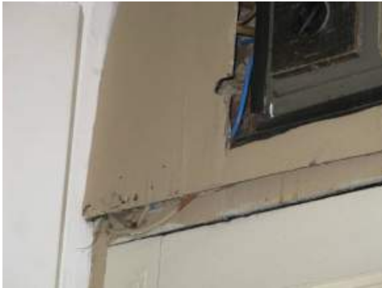
27-INSTALACION NO ORIGINAL
