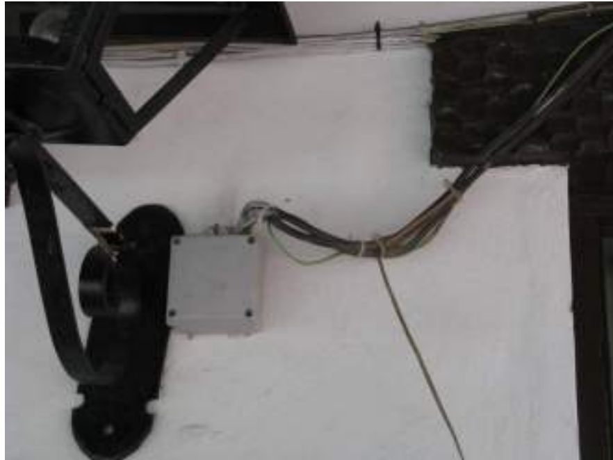
27-INSTALACION NO ORIGINAL-PERFORACIONES
