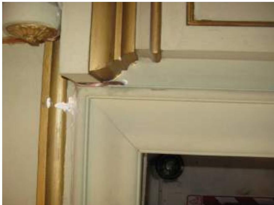
23-FALTANTE PARCIAL-INSTALACION NO ORIGINAL-PERFORACION
