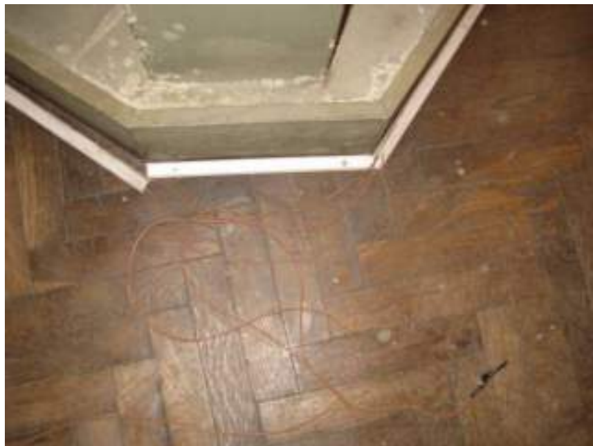
18-PA-INSTALACION NO ORIGINAL-PERFORACIONES
