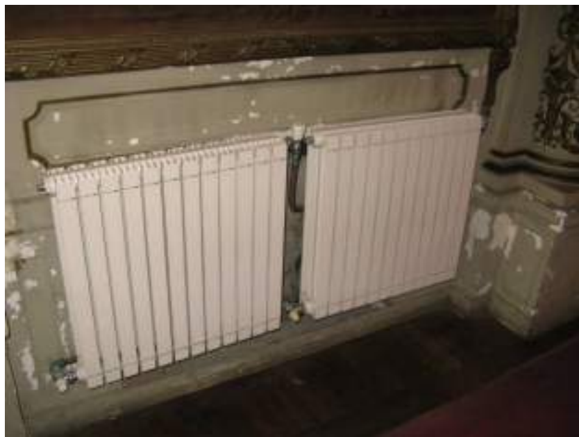
88-INSTALACION NO ORIGINAL
