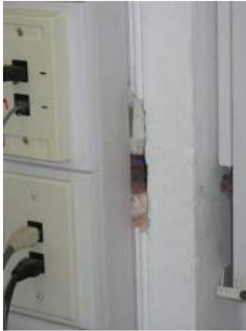
50-INSTALACION NO ORIGINAL-PERFORACIONES
