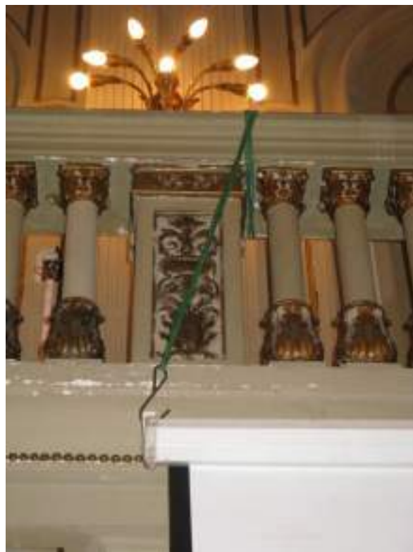
5-INSTALACION NO ORIGINAL-RAYADURAS
