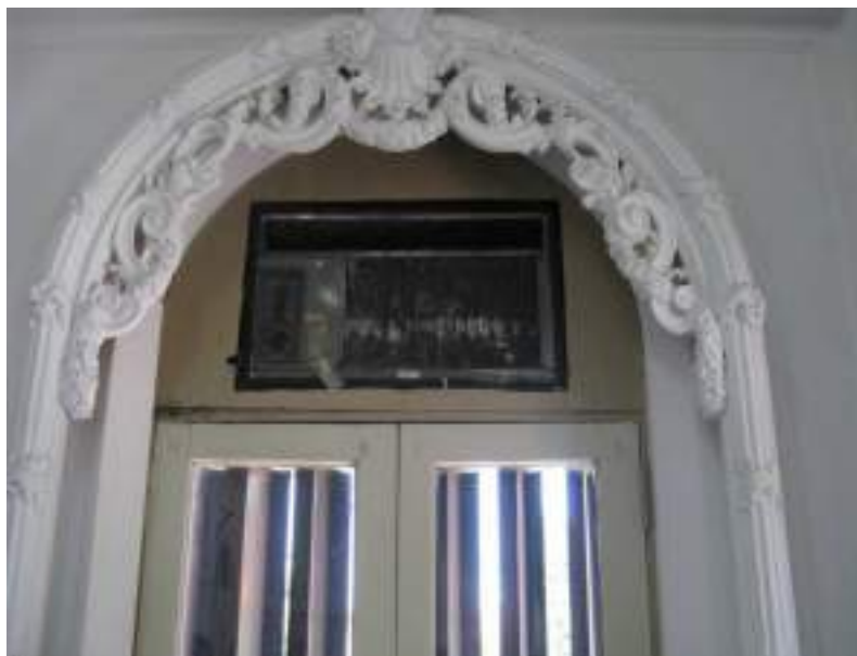
29-INSTALACION NO ORIGINAL
